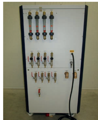
Laboratory cooler with multiple distributors on the device
